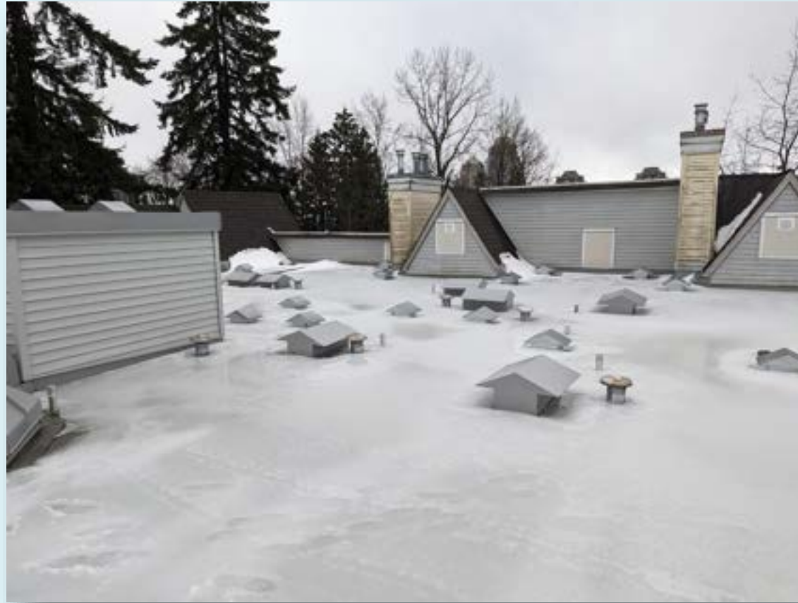
Greater Vancouver, December 24, 2022 (Credit: i3 Building Science & Consulting Inc.)
